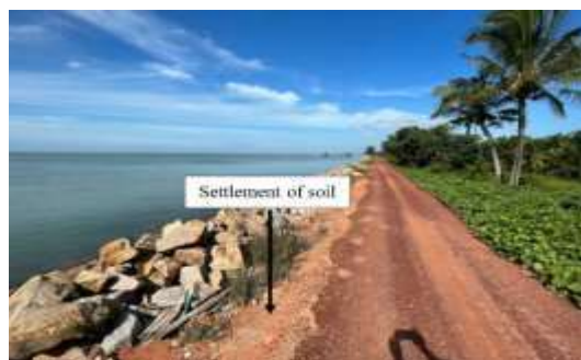
Fig. 1. Senggarang coastal embankment with severe seepage problem
